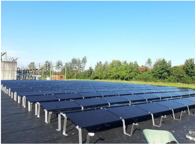
New solar plant at the Altgass substation: Modules with black frames were selected to blend into the local landscape.
